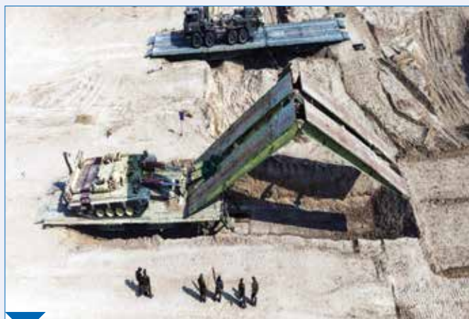
Exercise SARVATRA PRAHAR, Composite Crossing, Bridging, Breaching and Demolition Tasks, 10 Mar 26, Pokharan Field Firing Ranges, Jaisalmer.
