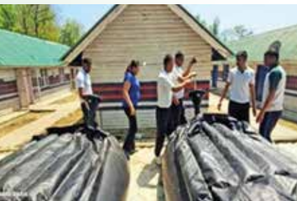
Bio Gas Plant, Srinagar Capacity 1-6 m 3 gas/ day Size 2-4 m dia digesters
